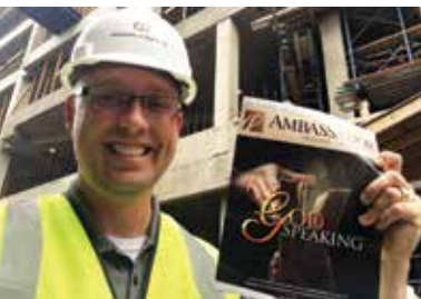
WASHINGTON D.C.: Progress! Another pic of construction underway for Museum of the Bible facilities (Washington D.C.). Thank you, Jeremy Burton!
