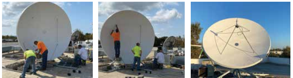
It's a little like an erector set, putting the new dish together. When it's all done, the signal is improved and the bits are flowing!
