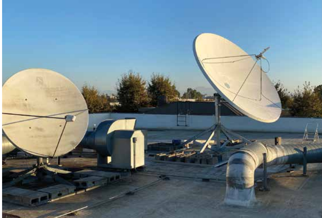
On the right: the brand new antenna! (The secondary dish in the left side of the photo is a Ku-Band antenna). The photos below show the step-by-step replacement process . . .
