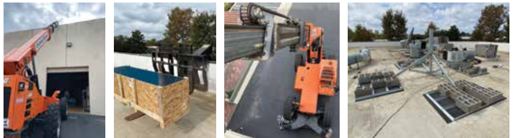
It starts with a high lift hoisting our new antenna mount on the roof. In no time, our new mount was put together.
